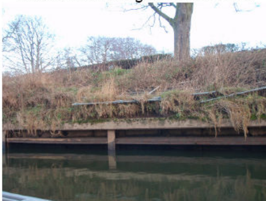
Upstream length: hole in bank covered with steel mesh fence
