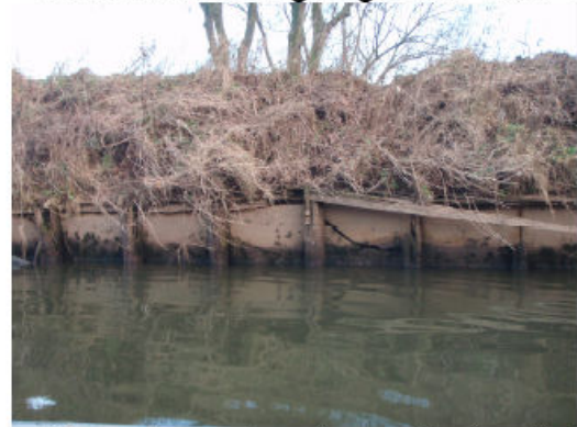
Downstream length: cracked wall
