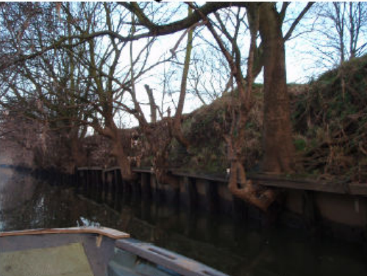
Downstream length: tree damage
