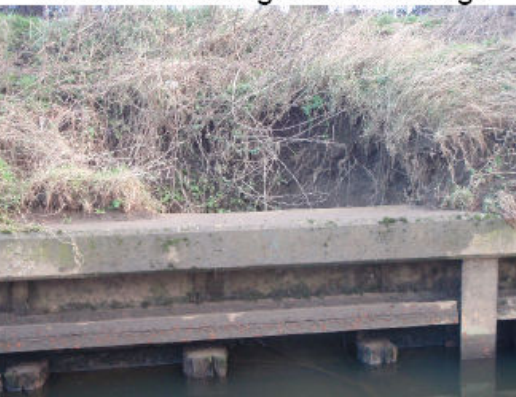
Upstream length: previous repair with hole in bank. Currently repairable
