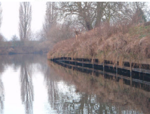
Upstream length: repairable length with failed length beyond
