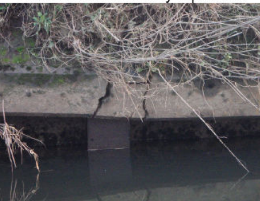
Upstream length: failed repair, replacement required
